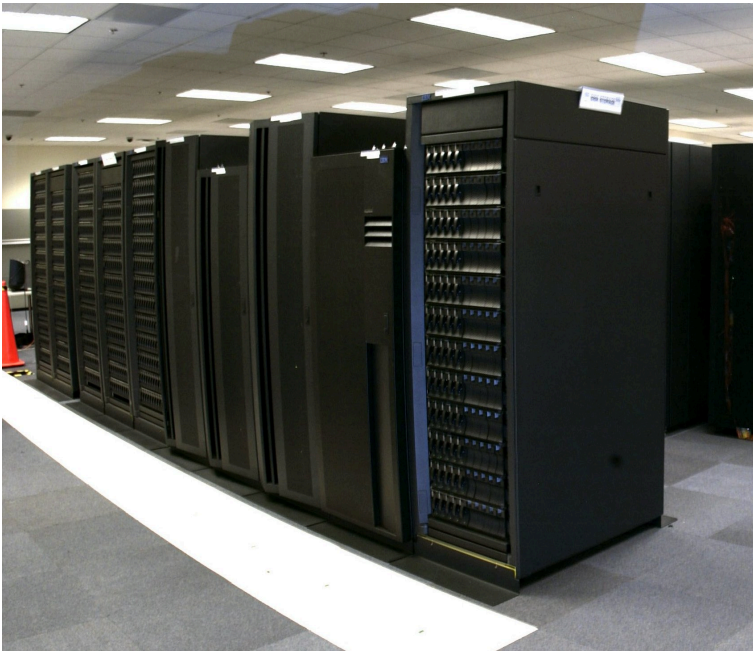
Figure 4.4: A Server Room in a Data Centre. A server is a powerful computer designed to manage network resources and provide services to other computers. Businesses and organizations use rooms like this, called data centres, to house servers that run their websites, store customer information, and manage company data. Image Credit: “IBM storage servers (1)” by NOAA Photo Library is licensed under CC BY 2.0, via Wikimedia Commons.
